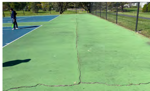
Cracks in tennis courts
