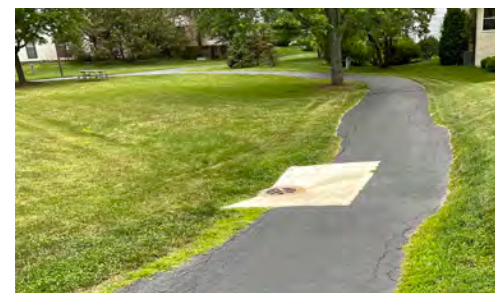
Drainage swale and inlet
