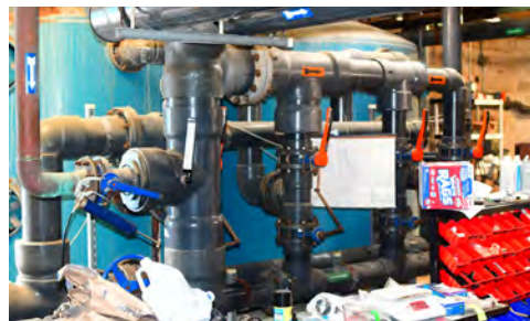
Mechanical pool plumbing
