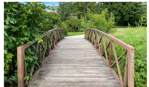
Pedestrian bridge in need of maintenance
