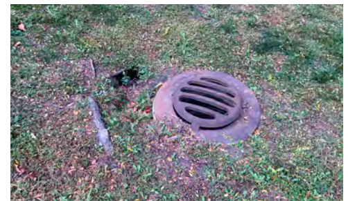
Drainage and erosion issue on west side of park
