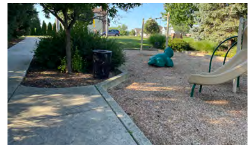
High curb and no ADA ramp
