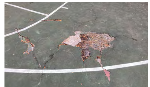
Spalling concrete at basketball court
